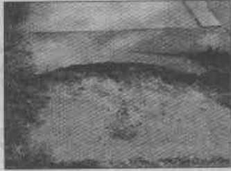
Homeowners are required to tell officials about hazards such as this.
