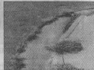
Grass growing in crevices along sidewalks is hazardous and speeds sidewalk deterioration.
